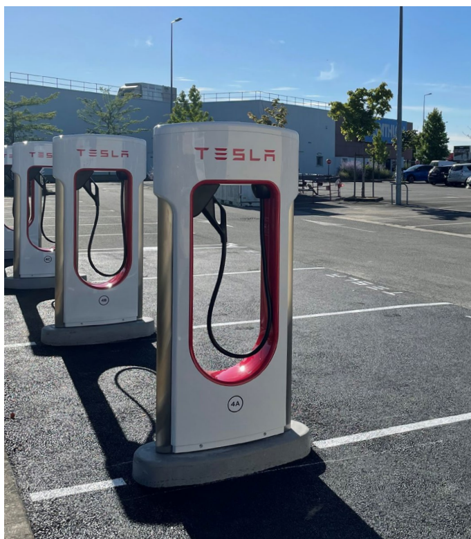
EV chargers on IREIT's Châtelleraut site (Decathlon store)
